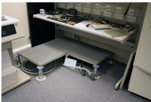
Raised Floor under CE work bench
